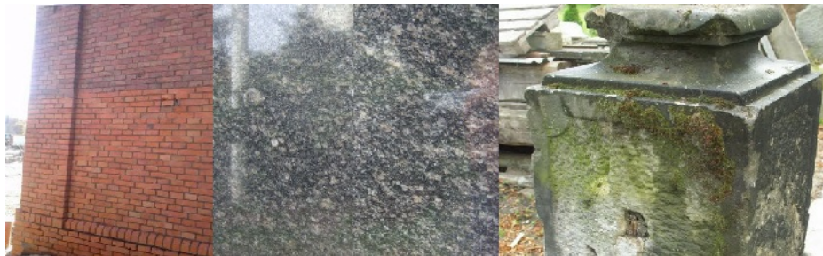
Fig. 1. Examples of defects of architectural details (volatile dusts, limestone blooms, soils of biological origin)
