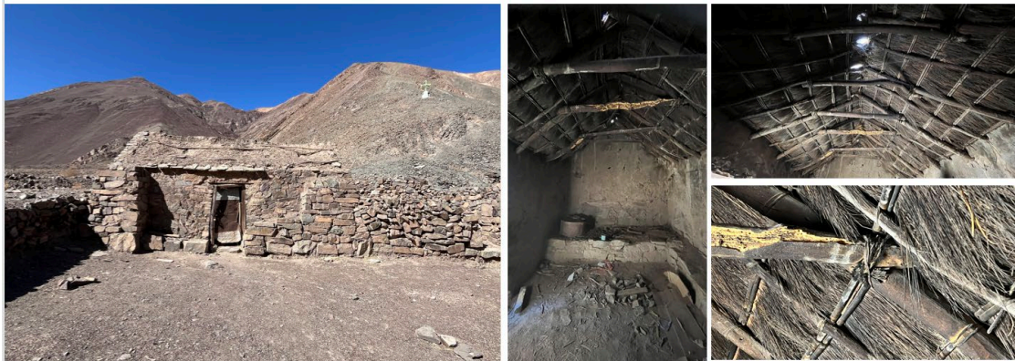
Figure 4. Exterior, interior and roof details of an Andean vernacular house in the town of Huatacondo.
