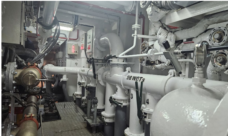
Fig. 2 Onboard ballast manually operated control valve system
