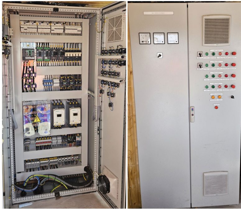
Fig. 3 Main electrical switchboard of the pontoon: open and closed states
