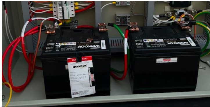
Figure 2: Storage battery connection
