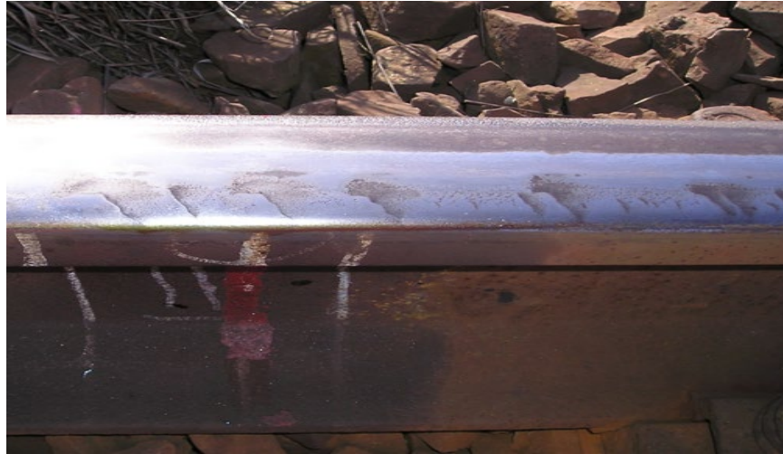
Fig. 1 Headchecking - rail under operating conditions
