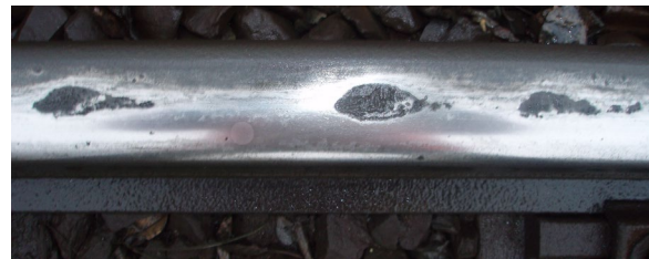
Fig 4. Shelling rail defect
